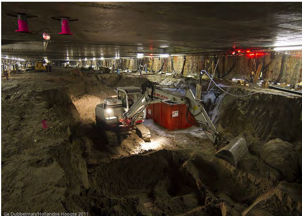
Figure: Impression of excavation deep part of the building pit under compressed air conditions.
