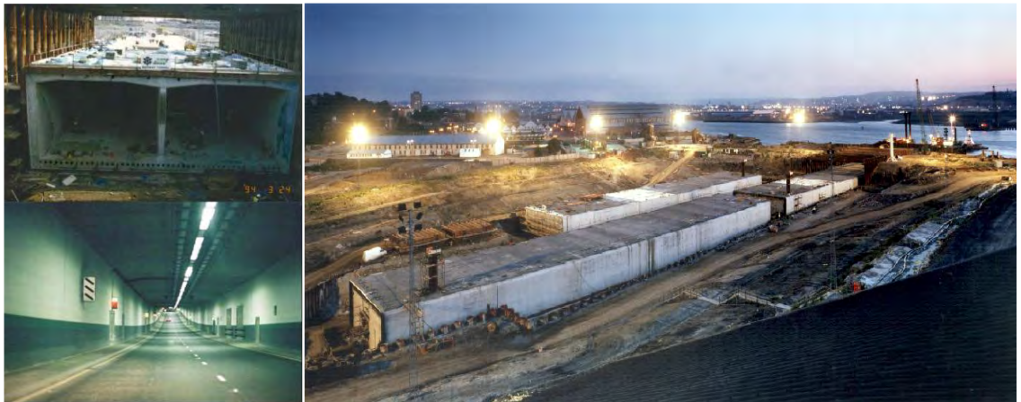
Figure: Medway tunnel under construction (top left, right) and completed (bottom left)
