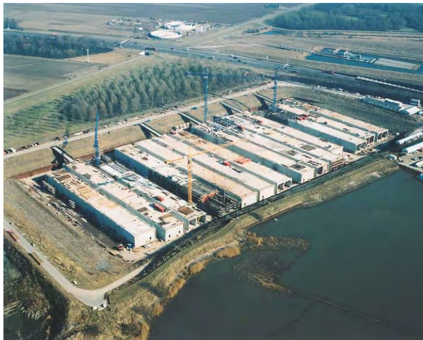
Figure: tunnel elements for crossing with river Oude Maas and Dordtsche Kil in construction dock
